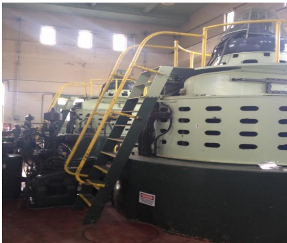
Figure 10: Grand Valley Power Plant Turbines
