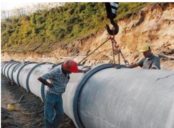
Figure 35: Concrete Penstock with Spun Rubber Ring Joints
