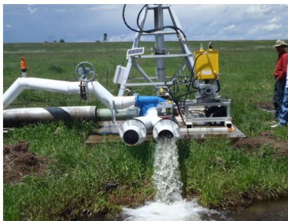
Figure 14: Bear River Ranch turbine
